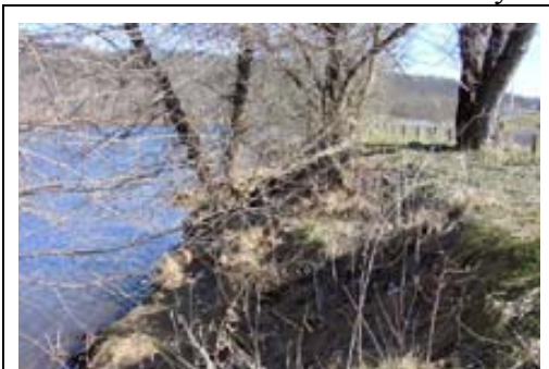
Sensitive area prone to erosion.
